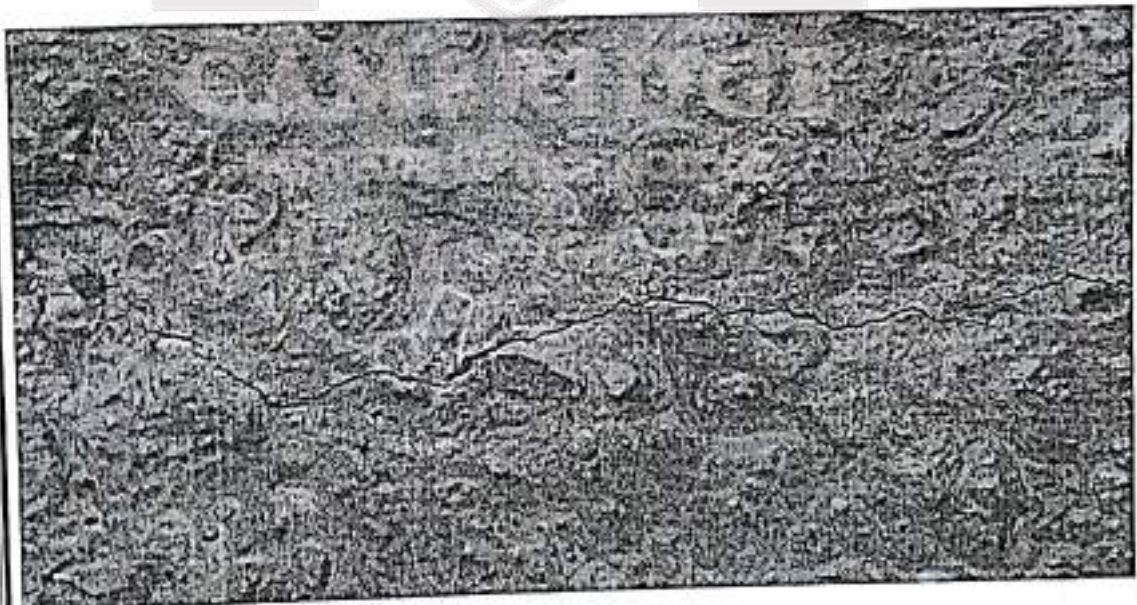
Figure: Autogenous shrinkage cracks
