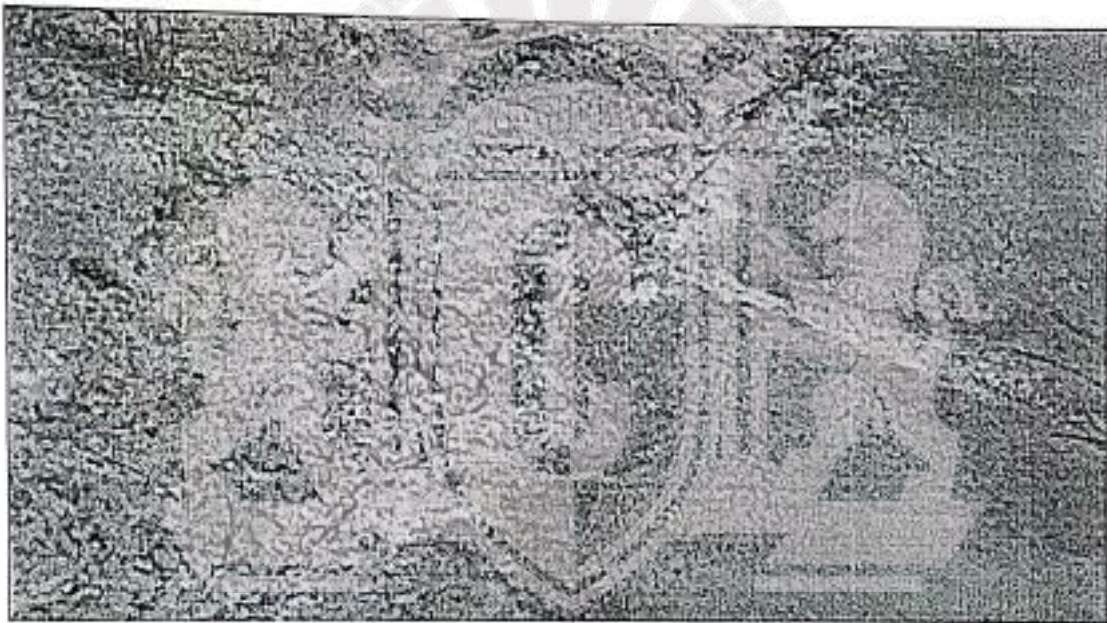
Figure: Salt attack on concrete
