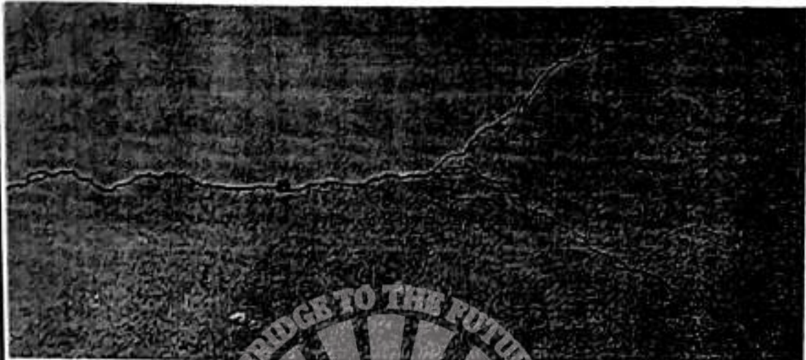
Figure: Plastic shrinkage cracks
