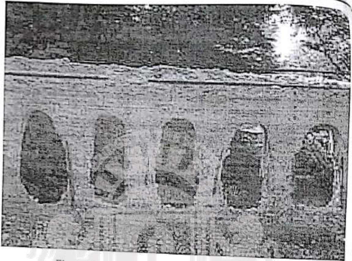
Figure: Damage of Bridge due to Freeze Thaw Cycles
