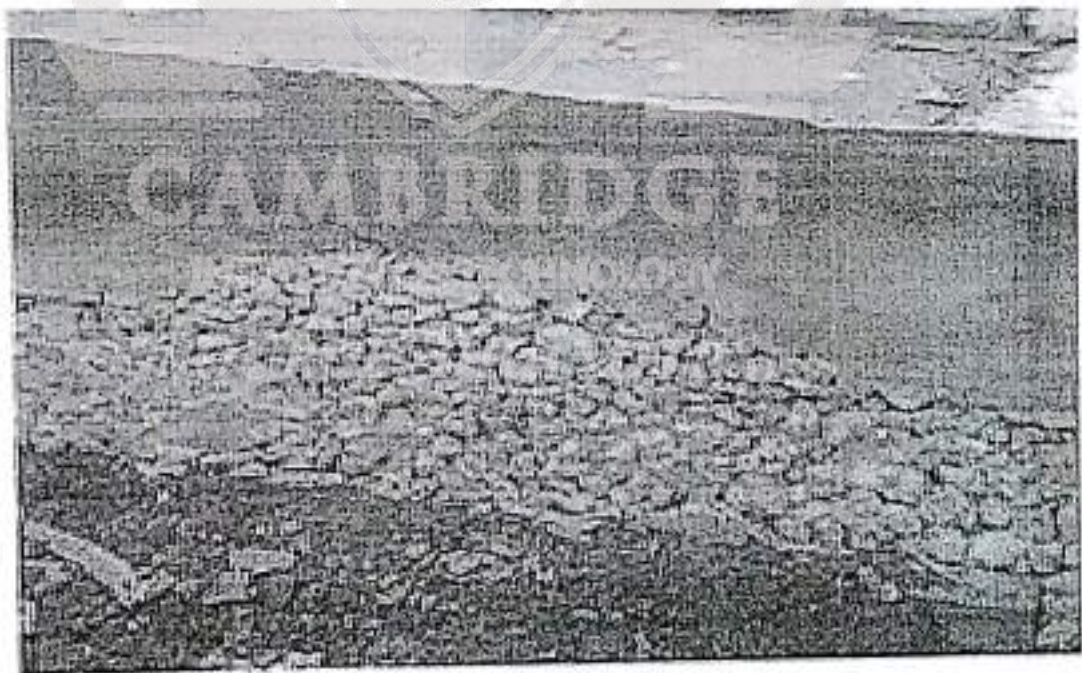
Figure: Exposed pockets of coarse aggregates
